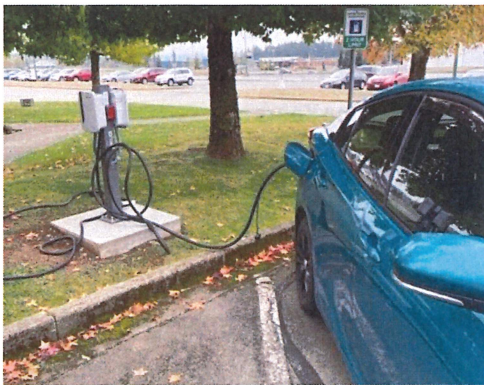
Port Alberni Campus EV Charging Stations
